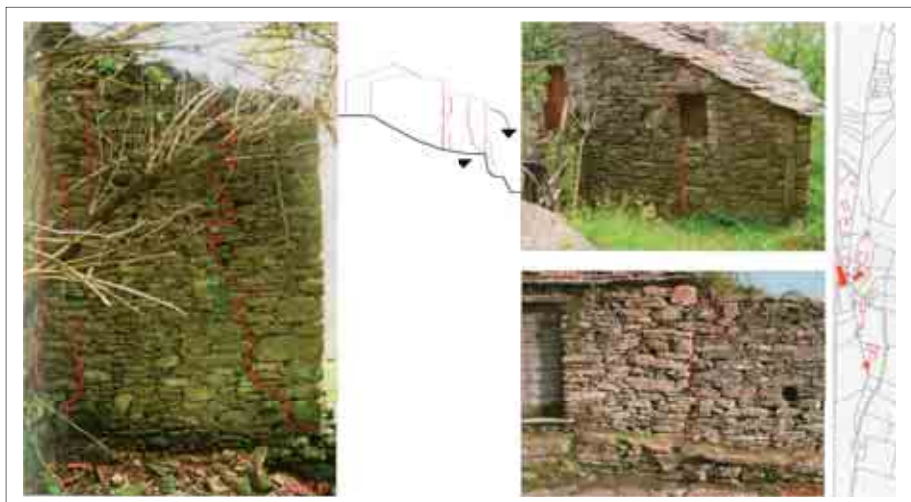
Fig. 4 Vergheto, structural decay after an earthquake (E. Massa)
