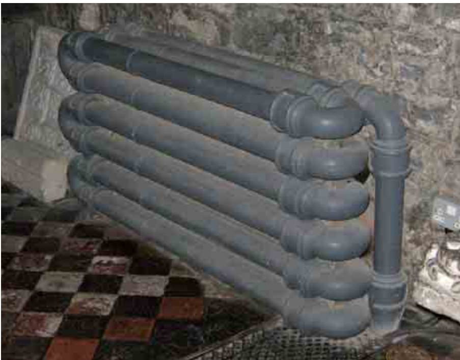
Fig. 4 St. Canice's Cathedral: the heating system
