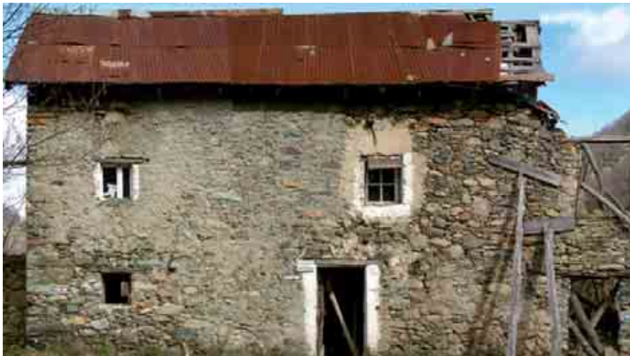
Fig. 5 Veirera, rural building partially collapsed
