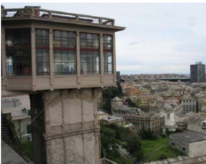
Figure 16. the Lift at Castelletto
